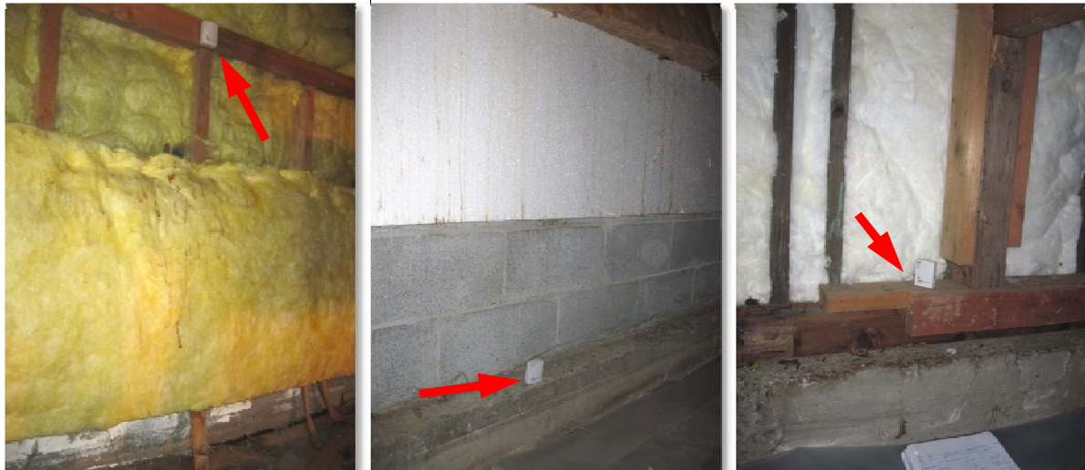
Figure 5. Temperature sensors installed near foundation walls to measure crawlspace air temperatures for one year.
