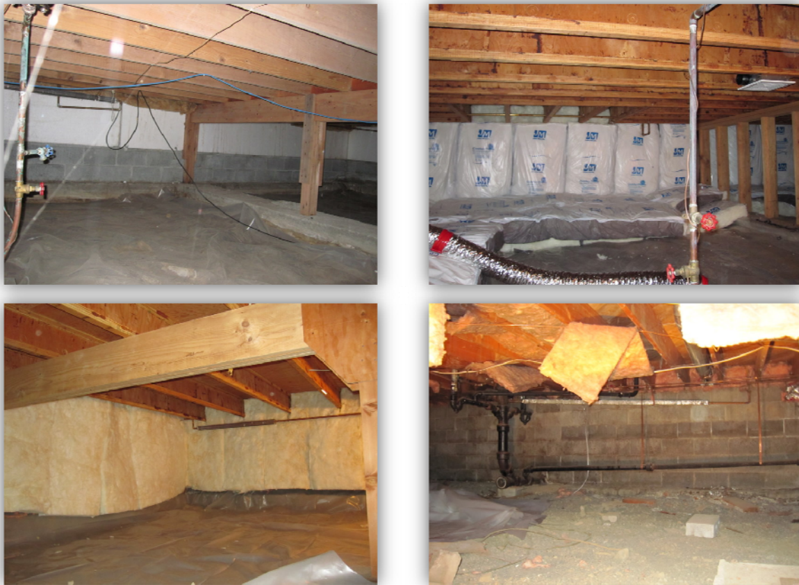
Figure 3. Typical crawlspaces involved in temperature study ranged from well-insulated to uninsulated conditions. The top left photo is representative of the most commonly encountered crawlspace insulation strategy, which includes one to two inches of rigid foam attached halfway down the stem wall. The top right photo shows an example of the R-38 fiberglass batt insulation draped down the stem wall with the ground insulation (the strategy under study). The bottom left photo shows R-19 fiberglass batt insulation draped down the stem wall. The bottom right photo shows an uninsulated stem wall and poorly insulated floor joists.
