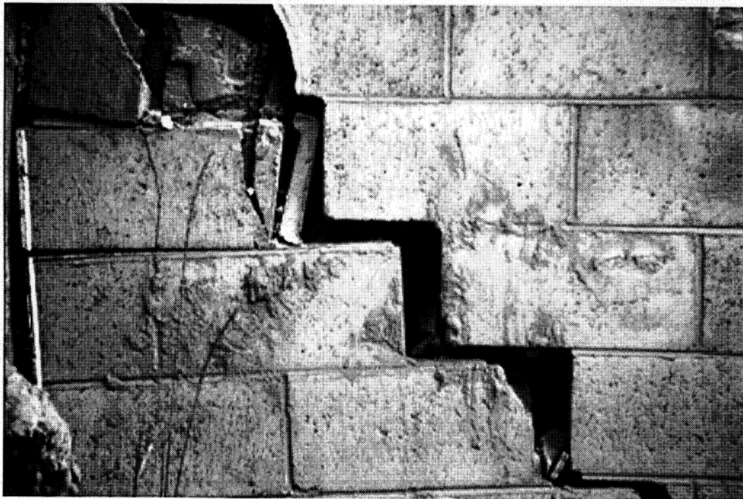
Figure 1.7 this is some of the foundation damage that thawing permafrost caused to the house above. Note that the cracks are wide enough for small animals to crawl through.
