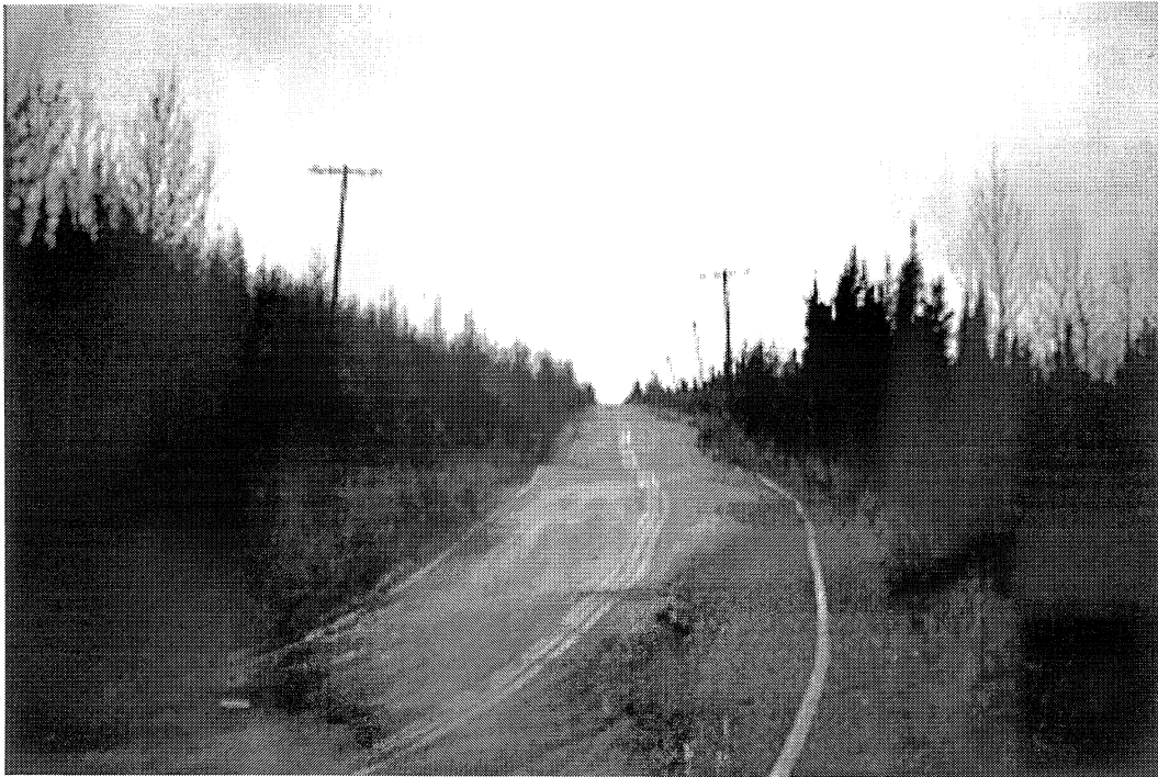
Figure A-4 Road traversing a permafrost area. Notice the “drunken” power poles along the road, as well as the undulating surface.
