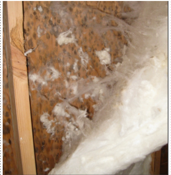
Figure 2. Mold on the sheathing behind the fiberglass on a wall with thin exterior insulation.
