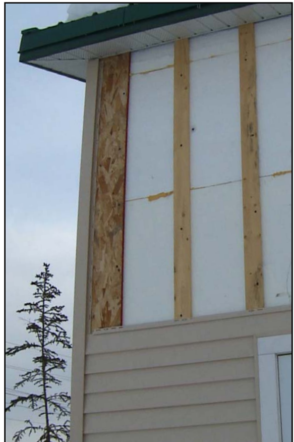
Image 34. Detail of wider furring on corner, allows for fastening to corner framing
