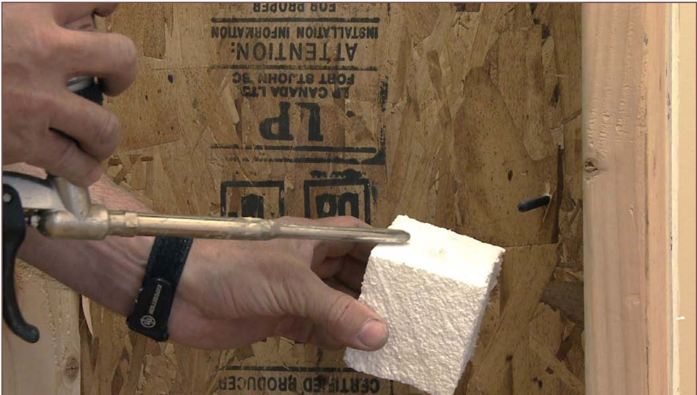
Image 31. Exposed fasteners inside the wall must be covered to prevent condensation
