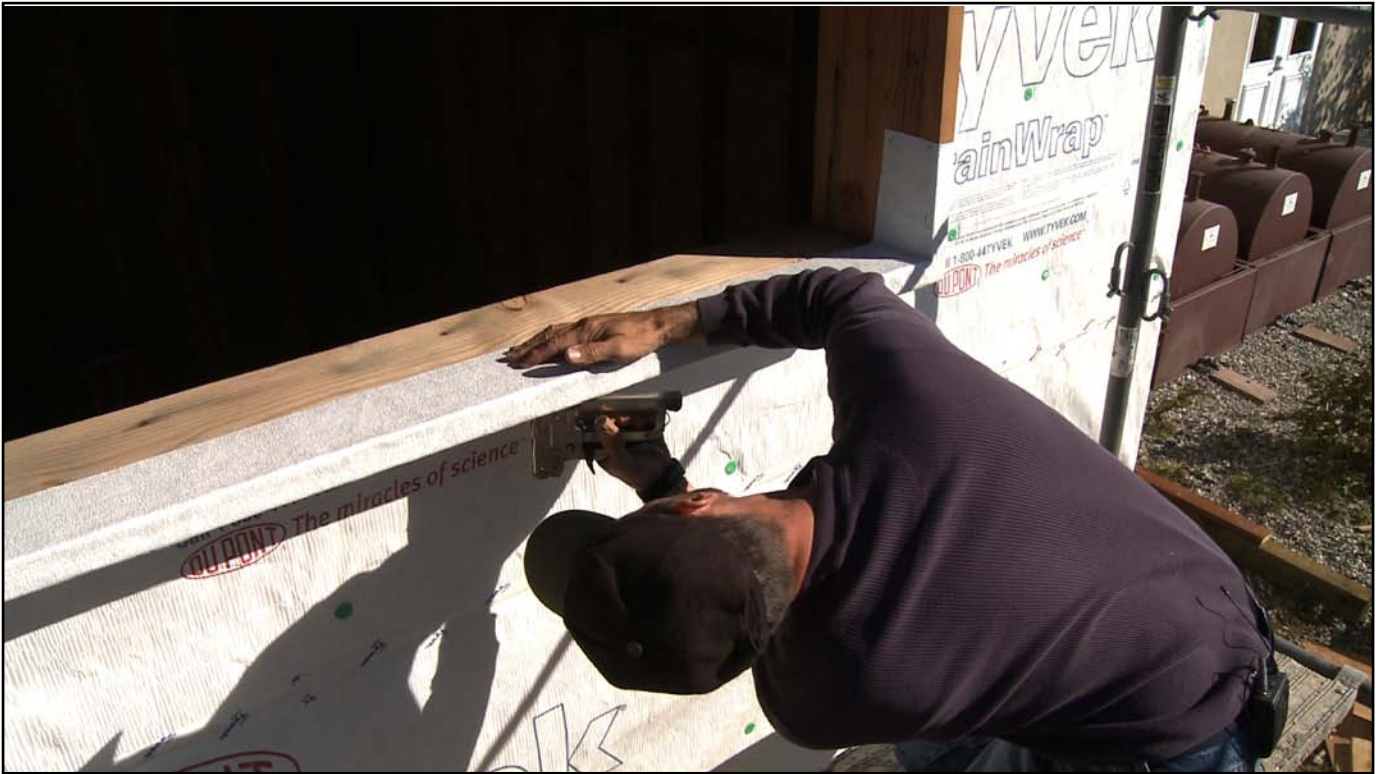
Image 10. Exterior window buck sill corner detail. Tyvek® FlexWrap™ (or similar product) must be stapled around edges
