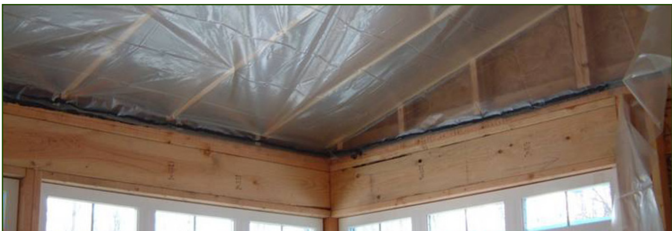
Image 24. Transition of interior ceiling vapor retarder to membrane strip on double top plates
