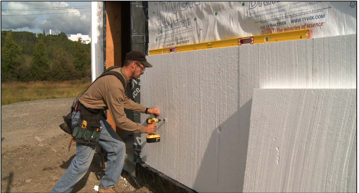
Image 25. Foam board is loosely attached to framing with a four inch sheetrock screw and a Wind-Lock® plastic washer
