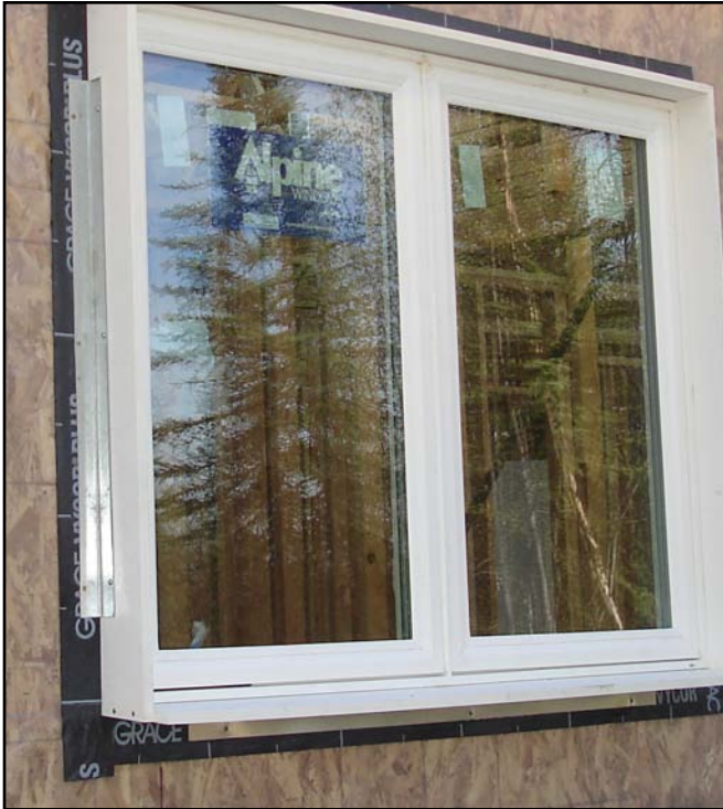
Image 13. Inset window with AZEK® jamb extension, attached to the sheathing using 2 inch x 2 inch light gauge galvanized flashing
