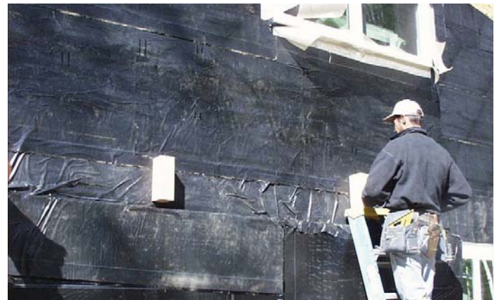
REMOTE wall under construction showing exterior vapor barrier, deck blocking & window detail.
