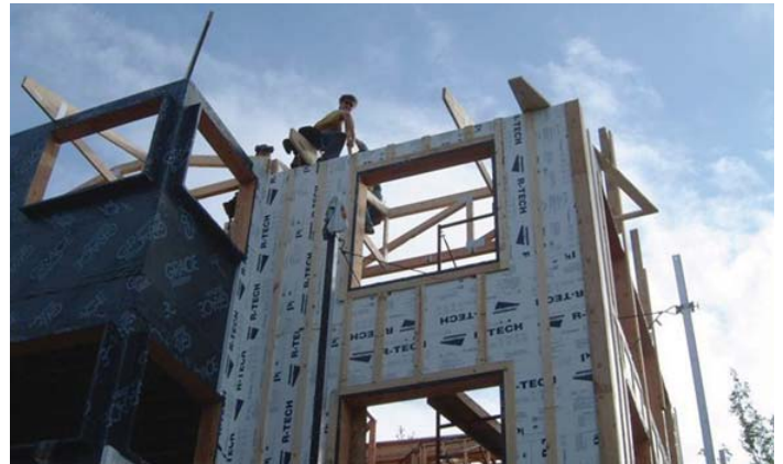
REMOTE wall under construction in Fairbanks, Alaska showing vapor barrier, insulation, window framing and furring in place for siding.
